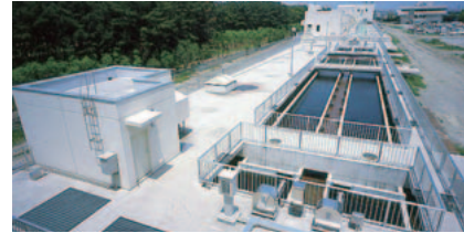
Matsugashima Waste Water Treatment Plant in Ichihara City (Chiba Prefecture, Japan)
